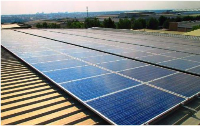
200 x 250W PV Panels
