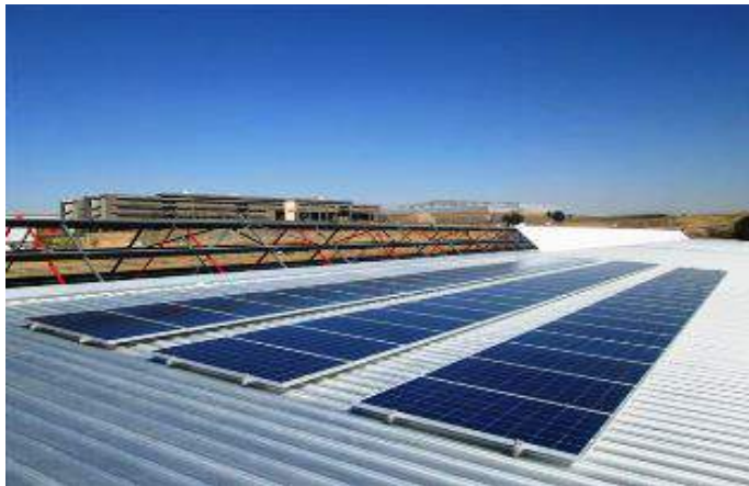
100 X 250W PV Panels
