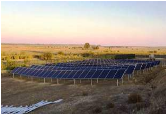
400 x 250W PV Panels
